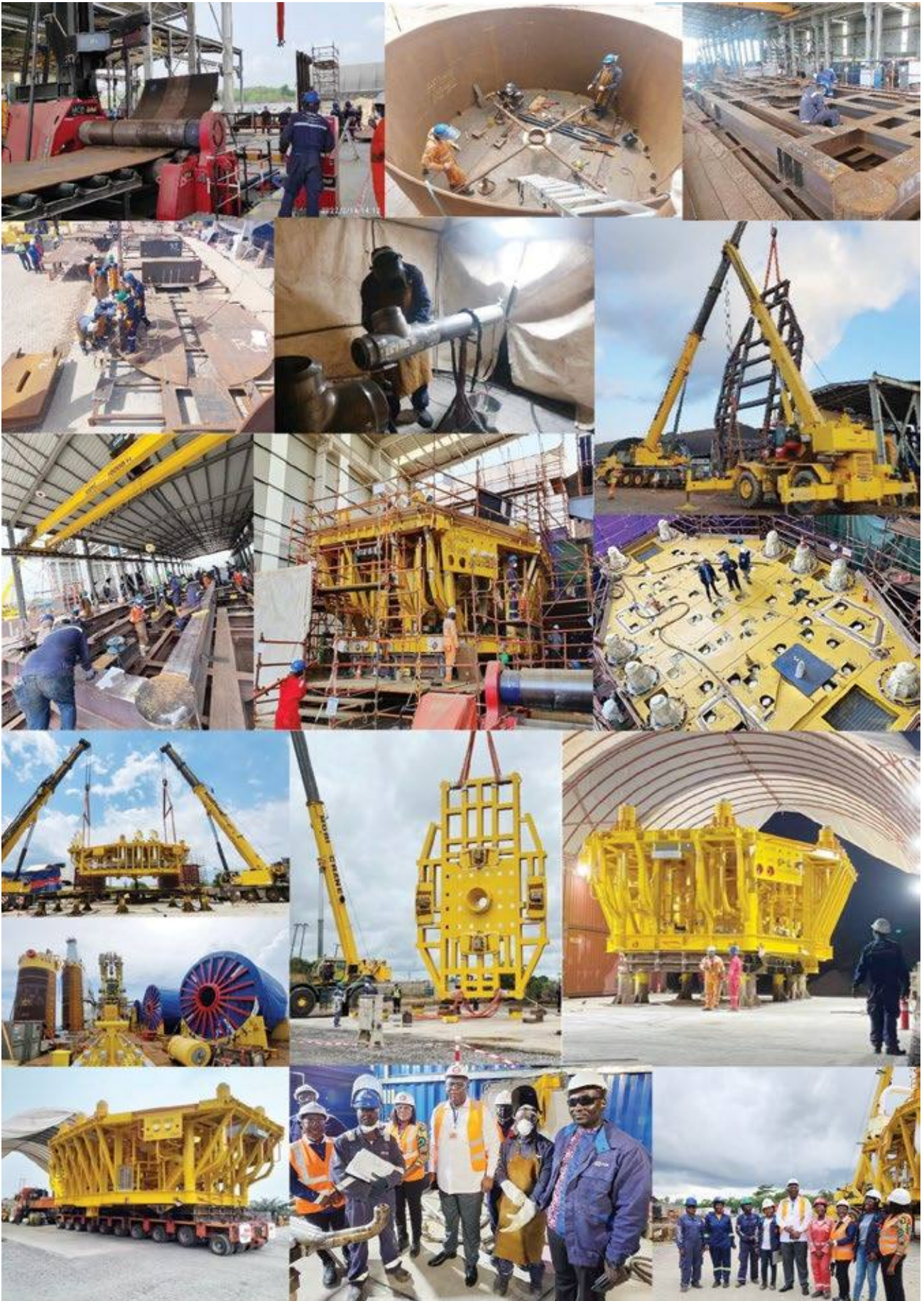
A picture gallery of the Orsam Yard during an inspection tour by the Commission during the fabrication of the P6 Manifold
